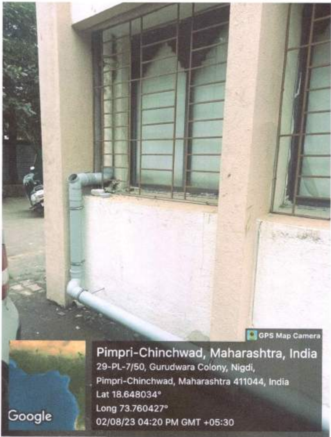
Geotagged picture of downpipe in rain water harvesting system at campus
