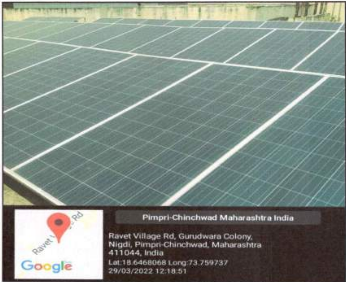
Geotagged Photograph of On grid Solar PV Plant at D Y Patil Educational Complex
